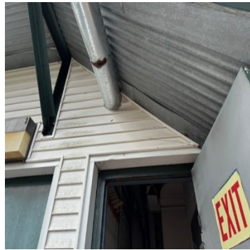
Rusted intake pipe
