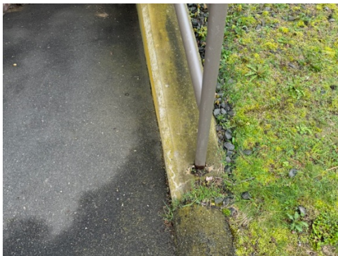
One metal handrail rotted at concrete embedment location
