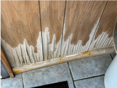
Interior wall damaged
