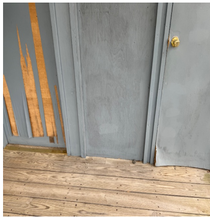
Interior door damage
