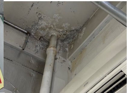
Water thru damaged concrete
