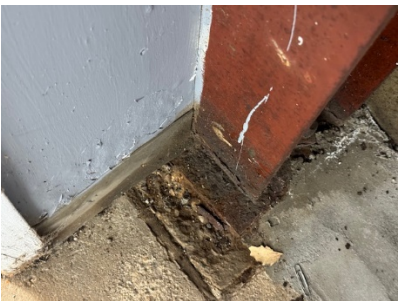
Interior column base rusting
