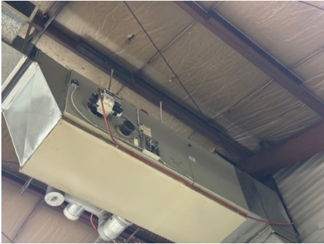
Hot air furnace
