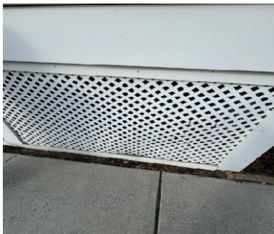
Broken & warped lattice
