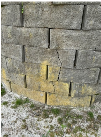
Crack in fnd wall under deck
