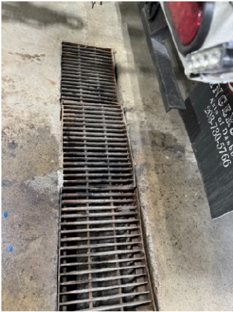
Floor grates not seated properly
