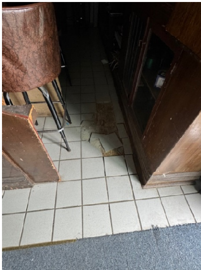
Broken floor tile
