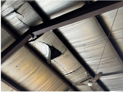
Damaged ceiling insulation
