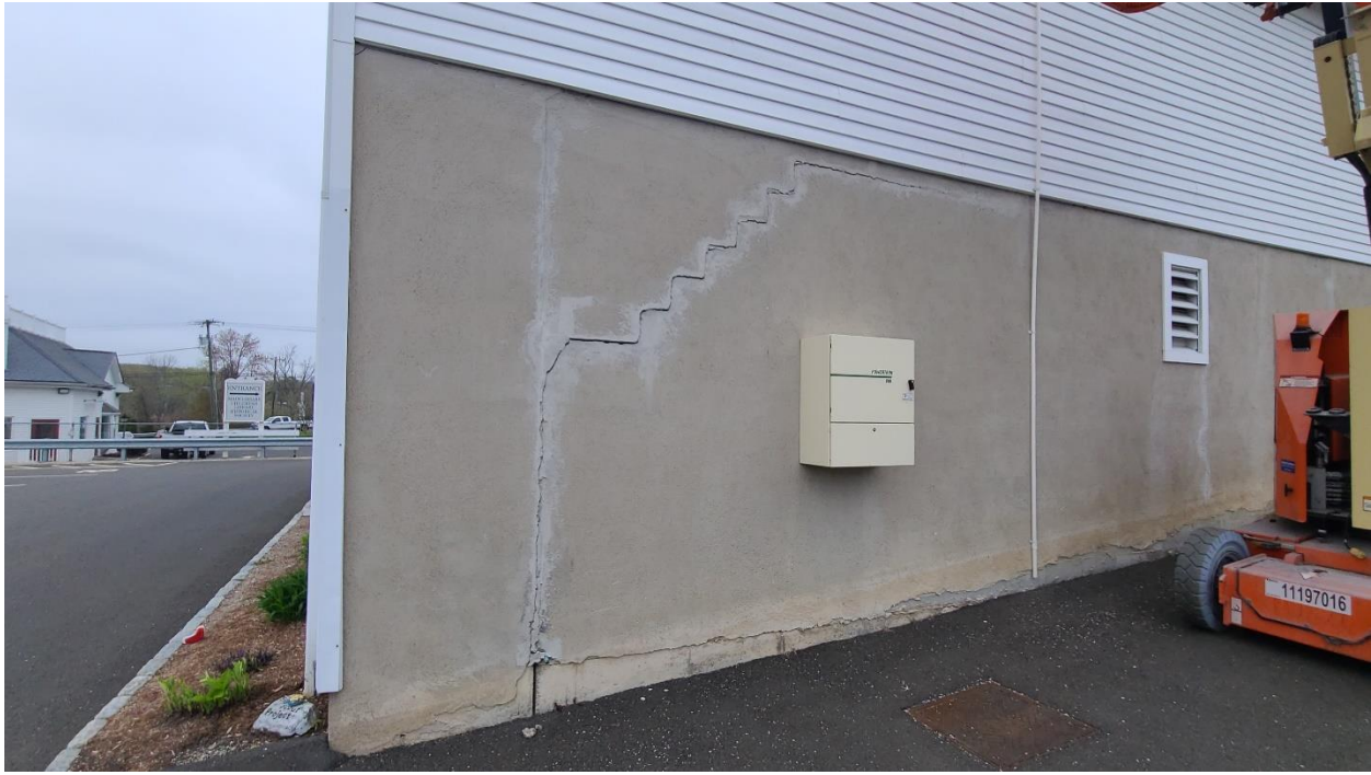
Photograph 1: Foundation crack - west wall
