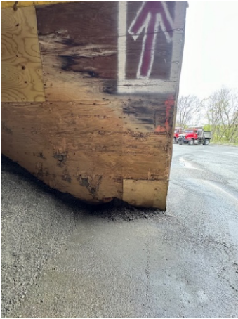
3/4-inch interior wall plywood damaged in few areas
