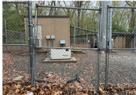
Broken gate panel
