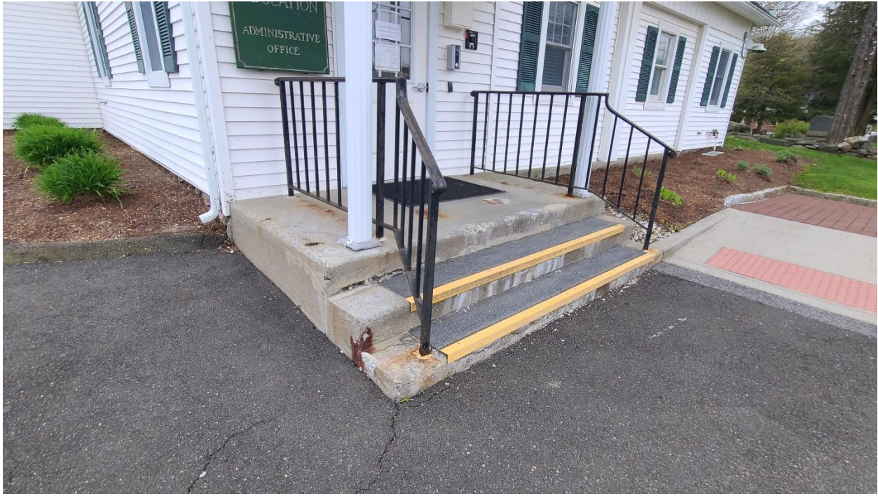
Photograph 1: Deterioration at front steps
