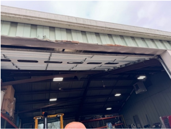
Overhead door header rusted
