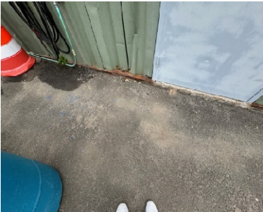
Exterior wall & sill plate rusted
