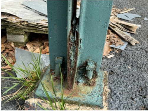
Corroded Column Base
