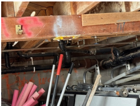
Column cap plate with no column in basement
