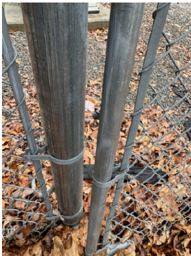
Broken bottom hinge of gate
