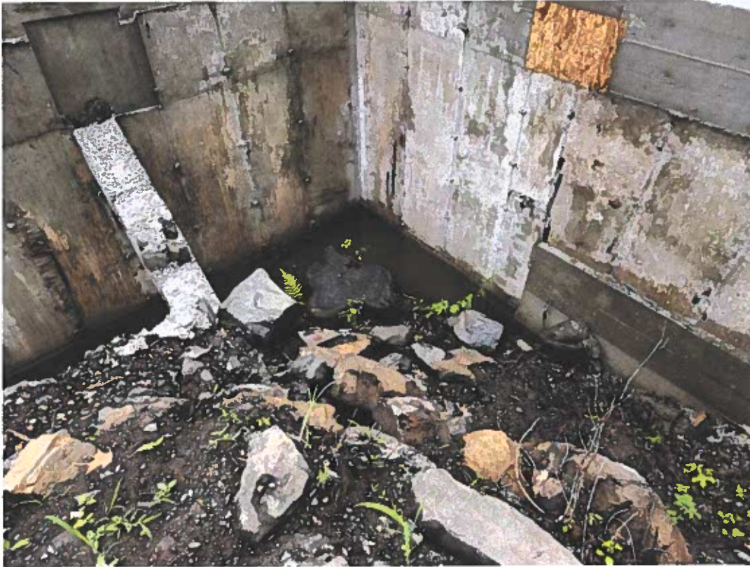
Photograph 4: Observed tree trunk/roots in excavation.
