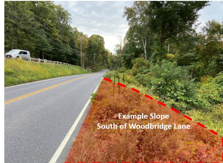
Figure 16: Steep Slope South of Woodbridge Lane
