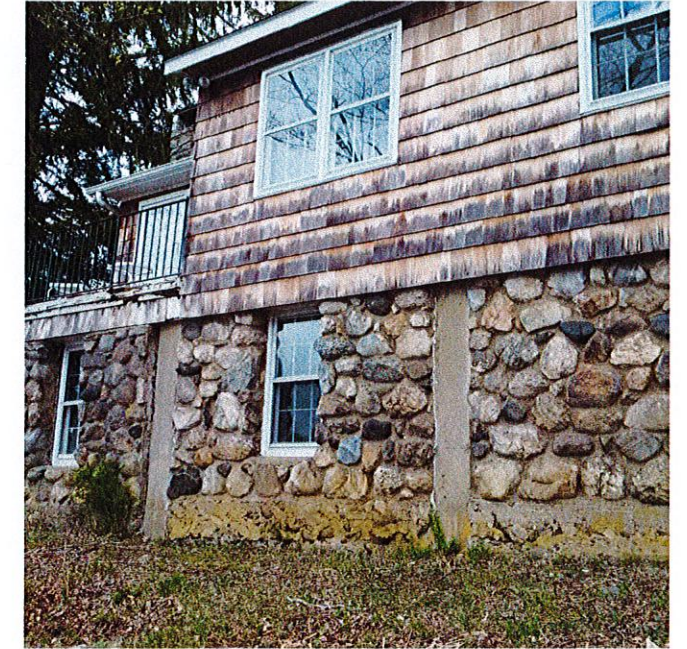
Pond view with failed terrace, 2021
