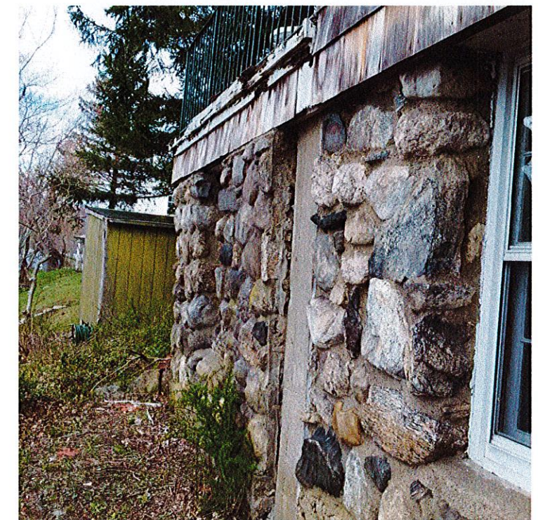
Enlarged pond view, 2021- damaged/rotted terrace
