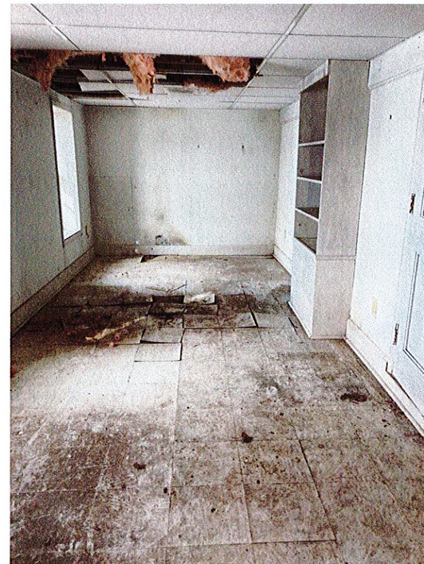
Damaged ceiling/basement due to terrace failure
