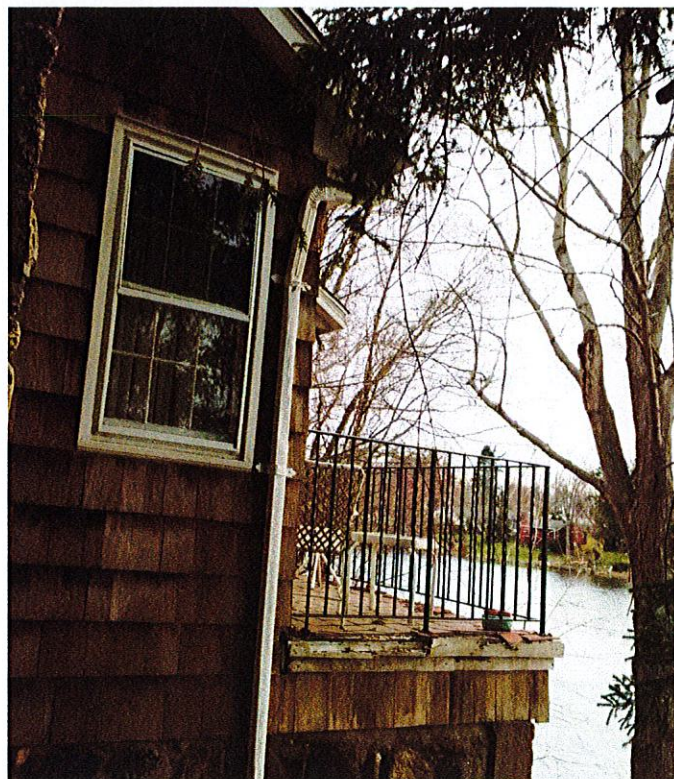
Damaged terrace from side of cottage, 2021
