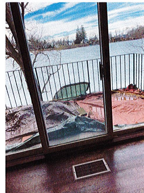
Damaged terrace from inside cottage
